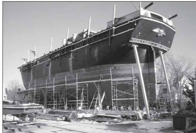
The Charles W. Morgan in dry dock awaiting renovations to take place over the next two years. Photo by Kristen Marshall
