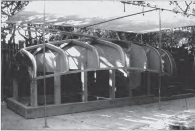
Sawn spruce frames attached to plywood mold sections in place on the strong back.
