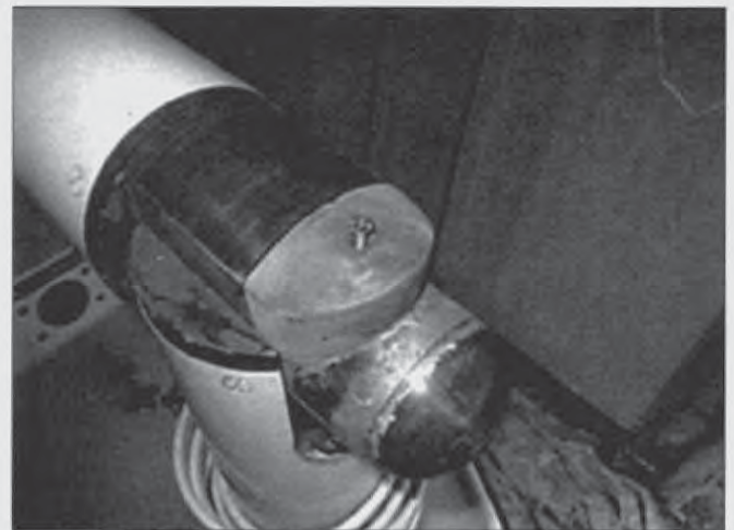
Plug in position, but would be attached to mast.
