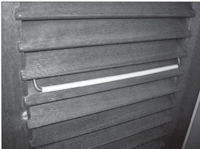
View of the attachment rod from the outside of the door.
