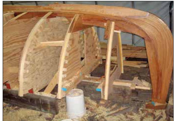
Forward end of the building jig showing the 80 lamination stem piece, keel joint, and forward cabin bulkhead and several station molds with attached floor timbers and laminated frames just prior to the start of planking.
