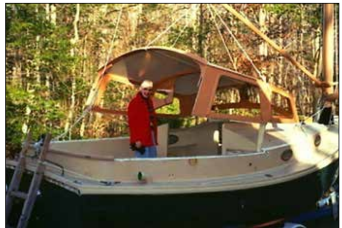
The epoxy/marine ply doghouse was assembled in our shop. Two people could easily carry it to the Muskrat where we picked it up with the gaff and slung it aboard. Dee is waiting to guide it in place.
