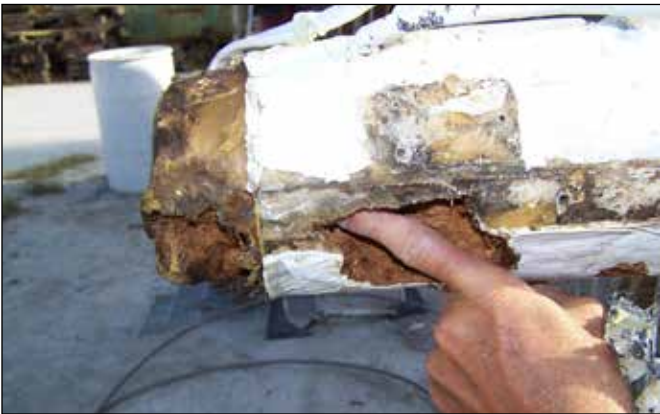
Rot at the top of the mast.
