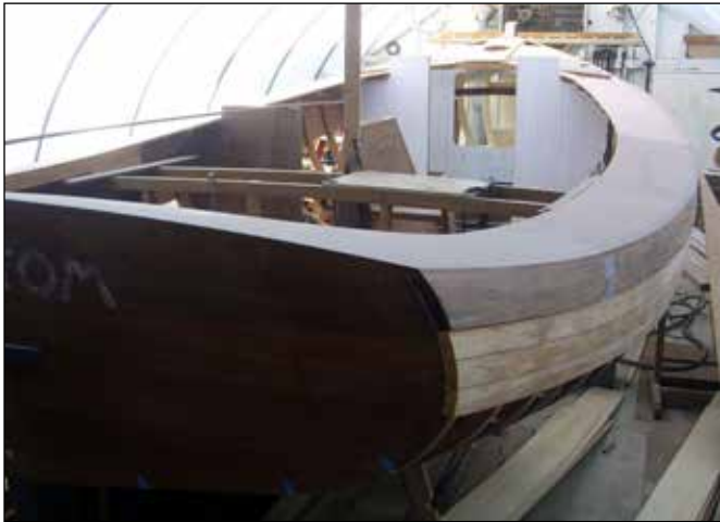
The sheer strake. Note the lower planking has been left unfinished at this point.
