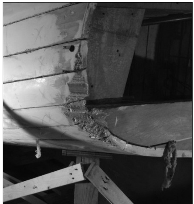
A ding in planks at the transom due to an owner mishap at the Barren Island Marina in Jamaica Bay about ten years ago will be repaired by scarfing new cypress planks.
