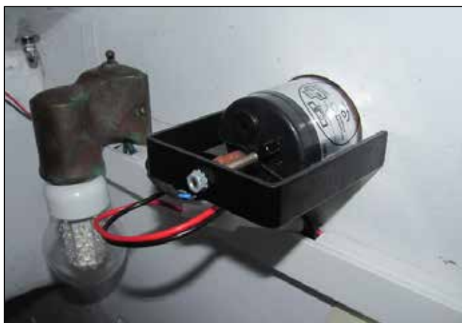
Figure 6. Depth finder display installed – inside.
