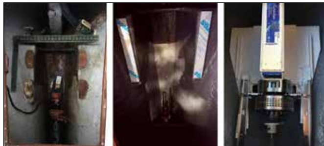
Left: The existing through-hulls needed to be sealed and the engine space cleaned. Center: Post cleaning and painting, the prop shaft was re-installed. Right: The motor mounted on its brackets and fitted into place.
