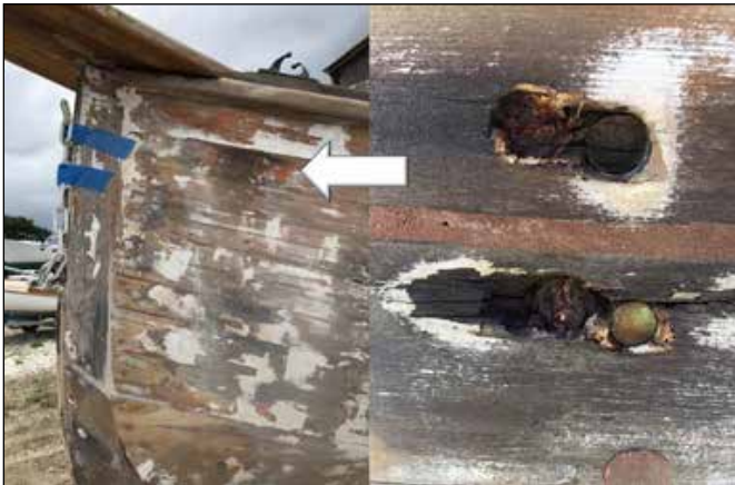
The taboo mixing of bronze and iron fasteners led to galvanic damage.
