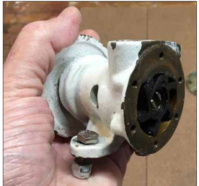
Figure 13. The saltwater pump was mysteriously unable to draw and pump cooling water.
