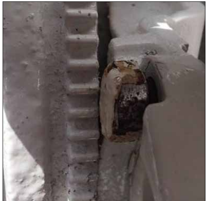
Figure 8. Release of one of the starter motor's mounting bolts required flywheel removal.
