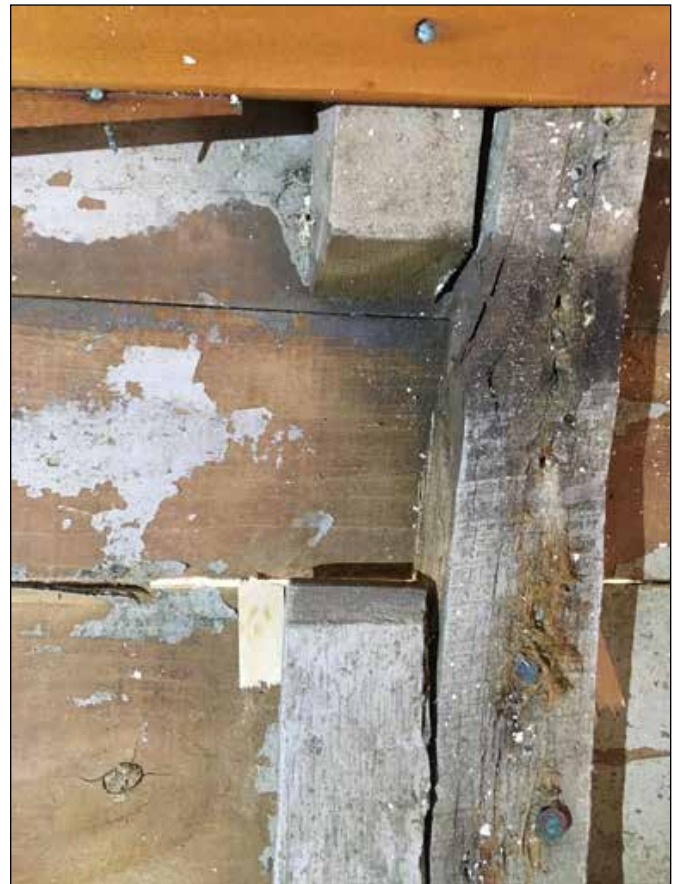
Figure 1 For some reason previous restorers left gaps in new, sistered ribs.
