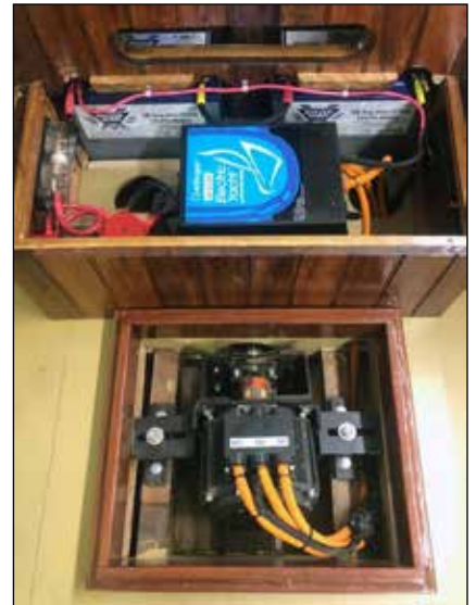
A direct drive, 24-volt electric motor from Electric Yacht was installed and powered with Battle Born LiFePO4 batteries.
